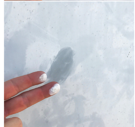
Painted surface oxidation
