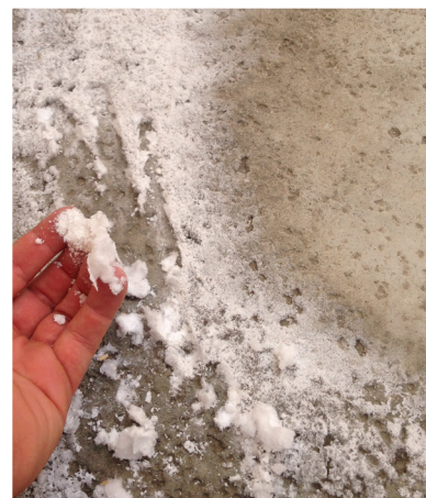
Use Efflo Process #1 Powdery Efflorescence on Concrete Eco Friendly Power Washing Palm Desert, CA
