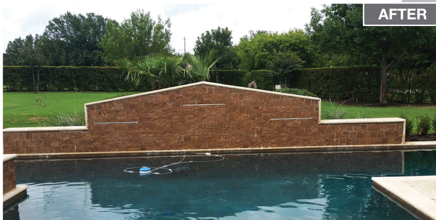
Efflo Process #2 Calcium Carbonate and Lime Run on Porous Brick Patriot Services Bedford, TX
