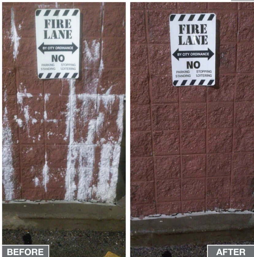
Efflo Process #1 Powdery Efflorescence
