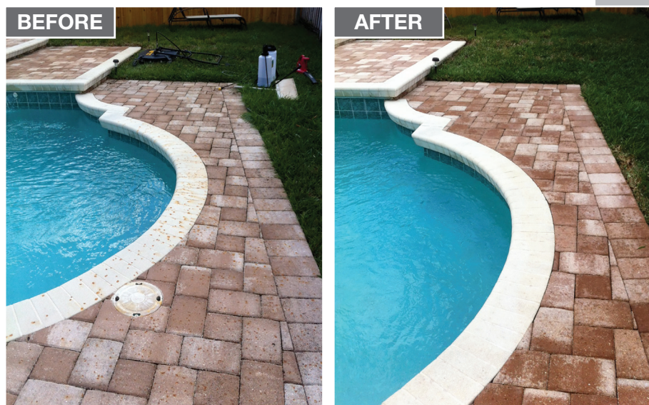
BARC Process #1 Fertilizer Rust Stains on Pavers
