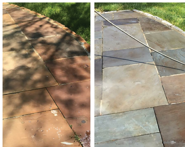
BARC Process #2 Irrigation Rust Stains on Tile
