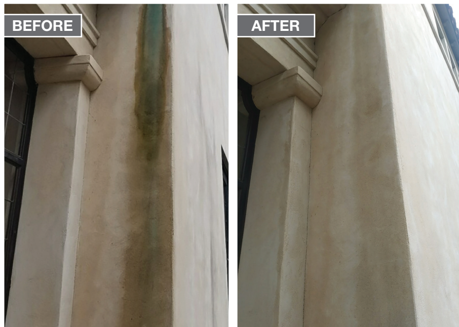
Efflo Process #2 Copper Stains on Stucco Squeaky Dan's LLC San Antonio, TX
