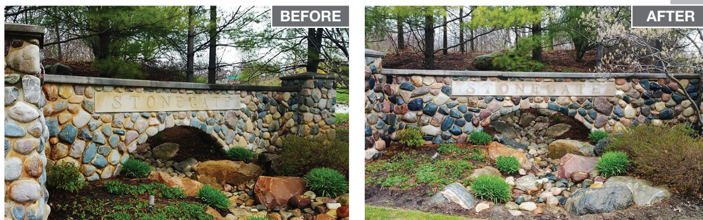
BARC Process #1 Light Rust Stains on Stone
