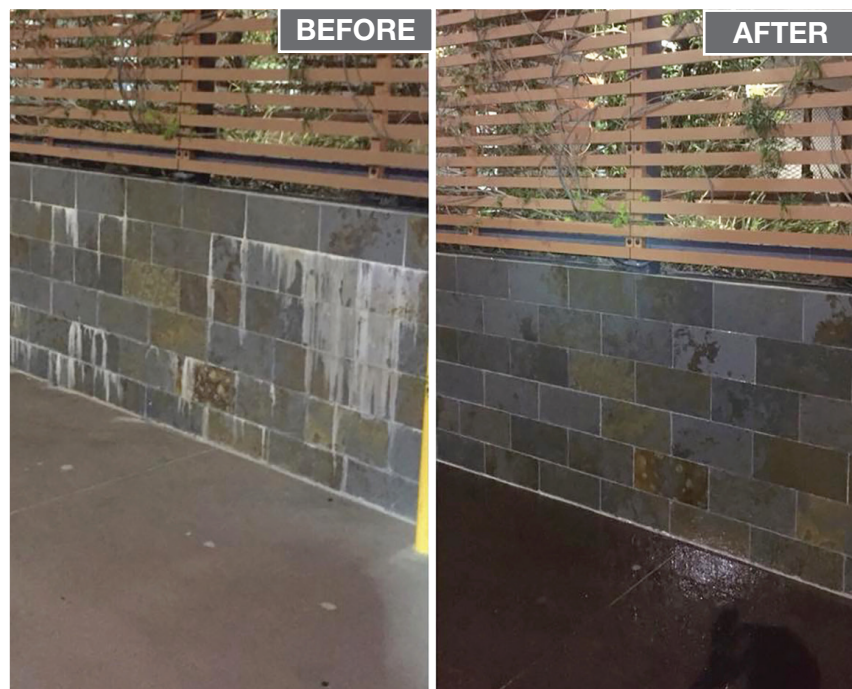
METHOD (A) Chart 7 Efflo Process #2 on Tile Poseidon Pressure Cleaning Queensland, Australia
